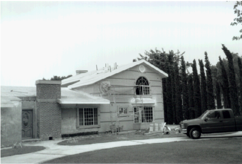
PICTURE 6. TYPICAL CONSTRUCTION ACTIVITY. THE GENERAL PLAN AND RELATED NOISE ORDINANCE WILL CONTINUE TO REGULATE THE HOURS OF OPERATION OF NOISE-GENERATING CONSTRUCTION AS WELL AS OTHER ACTIVITIES TO BEST PROTECT THE COMMUNITY.
