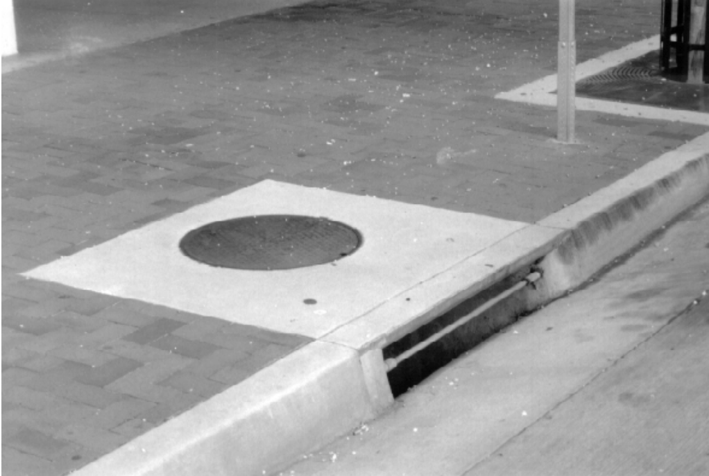
PICTURE 10. ORDINARY STORM DRAIN INLET. BESIDES ADDRESSING STREETS, THE CIRCULATION ELEMENT ALSO ESTABLISHES A FRAMEWORK FOR MAINTAINING AND, WHERE NEEDED, IMPROVING STORM DRAINS AND OTHER INFRASTRUCTURE.
