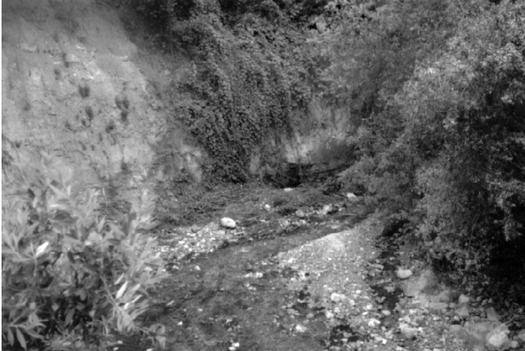
PICTURE 9. VIEW OF THE UNDEVELOPED PORTION OF WALNUT CREEK, LOOKING WEST FROM THE BRIDGE SECTION OF THE CURVE THAT SERVES AS THE TRANSITION FROM SOUTH REEDER AVENUE TO EAST PUENTE STREET. THE PICTURE SHOWS THE EFFECTS OF FLOODING AND EROSION IN THIS SENSITIVE AREA, PROBLEMS THAT THE SAFETY ELEMENT SEEKS TO COUNTERACT AND REMEDY.
