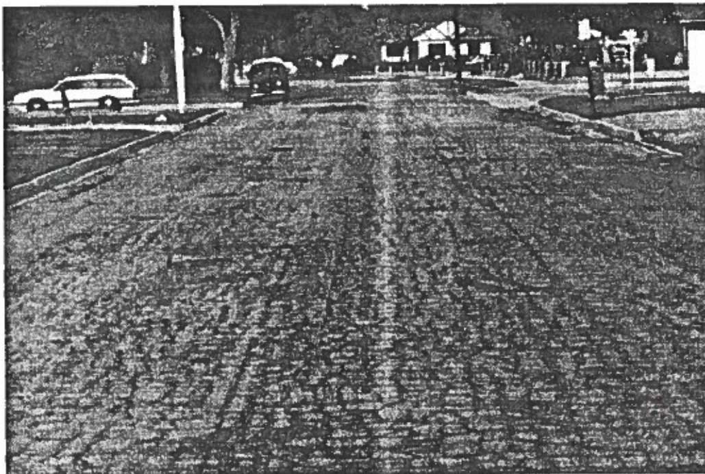
PICTURE 11. TYPICAL DETERIORATING STREET. MANY PUBLIC STREETS ARE IN NEED OF RECONSTRUCTION OR RESURFACING, A FACT THAT THE CIRCULATION ELEMENT RECOGNIZES AND DEALS WITH.
